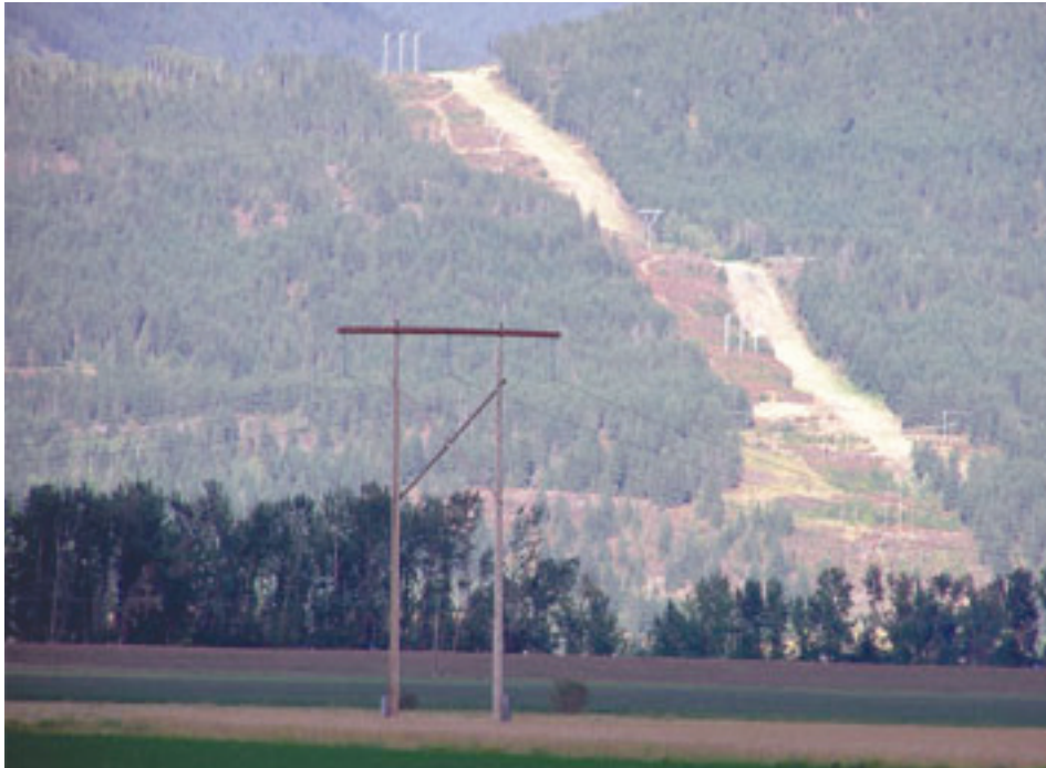
Transmission lines accompany the development of all private hydro projects. Photo by Gary Diers.
