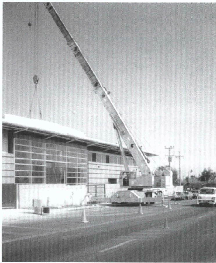
Installation of the bridge crane at Escondida Technical Institute, in Antofagasta, Chile.
